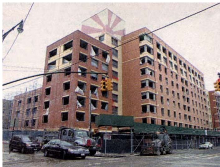
Palacio del Sol is under construction on Melrose Avenue between 156 th and 157 th . - Magnusson Architecture and Planning PC
